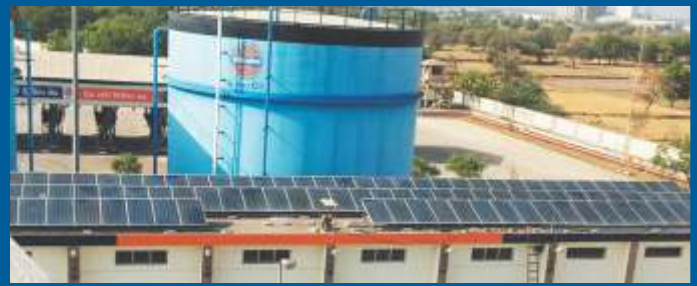
Installed Capacity- 225KWp Location- IOCL, Gujarat
