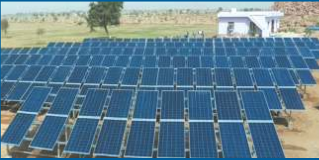
Installed Capacity- 100KWp Location- Rajasthan
