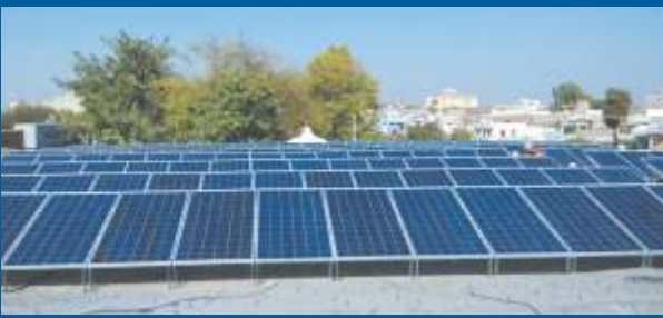
Installed Capacity- 280KWp Location- Indian Railway, Rajasthan
