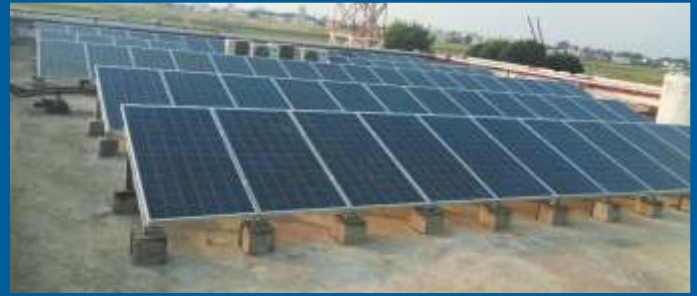
Installed Capacity- 150KWp Location- Airport Authority of India, Rajkot
